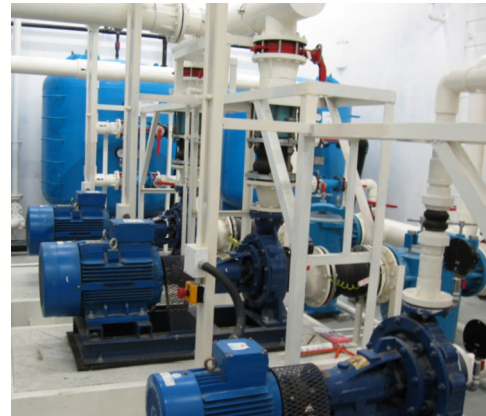
Filtration plant of swimming pool
