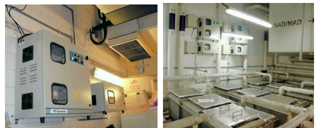
CR-400i used at the garbage room and grease trap room of IFC
