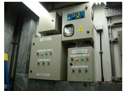
CR-200i used at TST East station of MTRC
